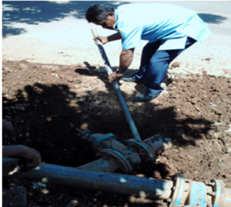
Gambar 4.3: Kebocoran Pipa Logam Akibat Korosi (Rumah Belajar, 2009)
